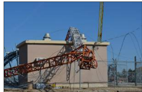
REFERENCE - FALLEN ANTENNA TRUSS
